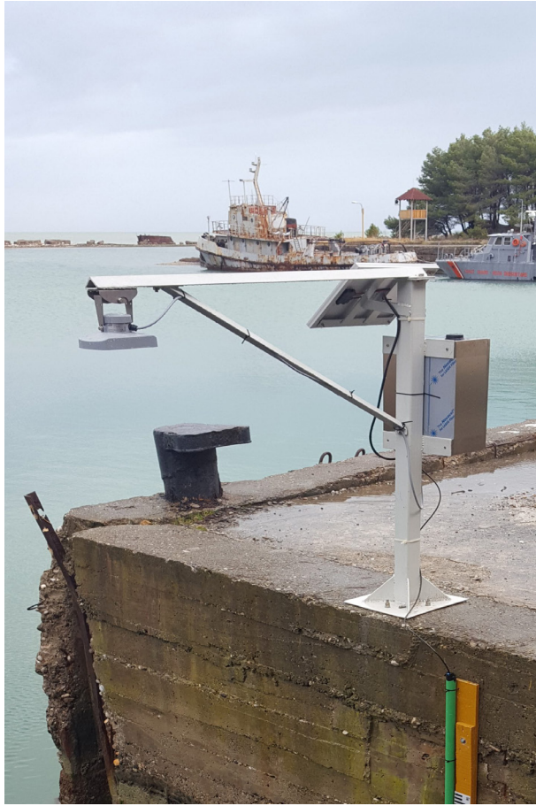
Figure 2: View of the Durrës Tide Gauge at Cape of Pal (Kepi i Palit)
