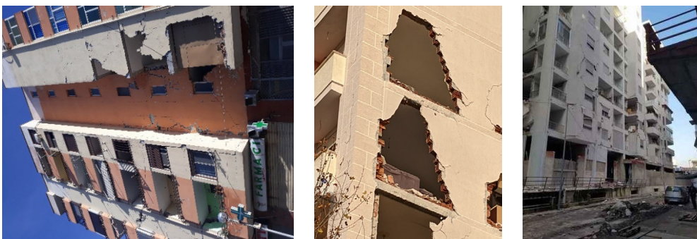
Figure 4: Buildings with non-structural damage
