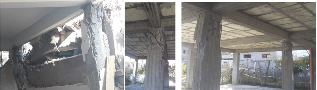
Figure 2: Buildings with major structural damage.
