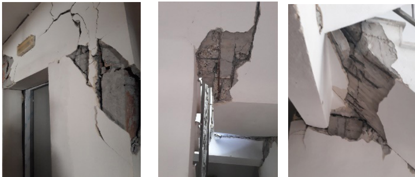
Figure 2: Damages in interior staircase in school buildings during visual inspection in Durres
