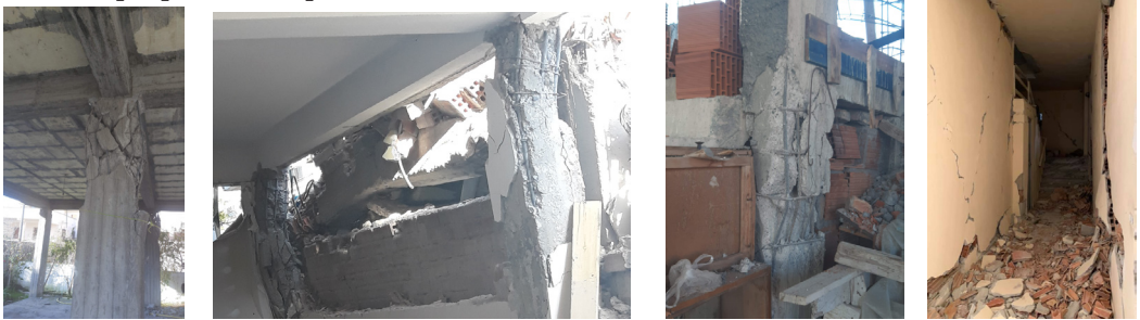
Figure 1: Damages in a school building in Durres
