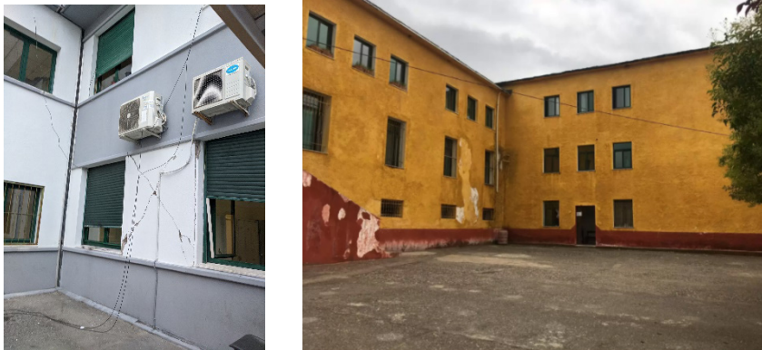
Figure 4: Exterior damage in school building in Durres
